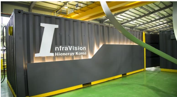
<Energy Storage System40 pt>
